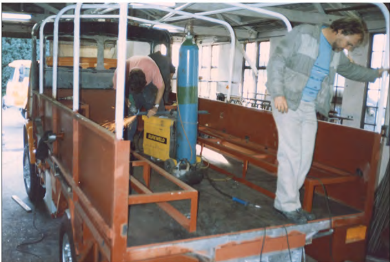
Timber floor and seat frames have been fitted. Underfloor locker for tent poles is in place. Mounts for spare springs are welded on each side. The hard front of the passenger compartment has been secured in place sitting on hard rubber mounts. Bill Preston (workshop manager) is standing, and Matt Hollingsworth is on the grinder.
