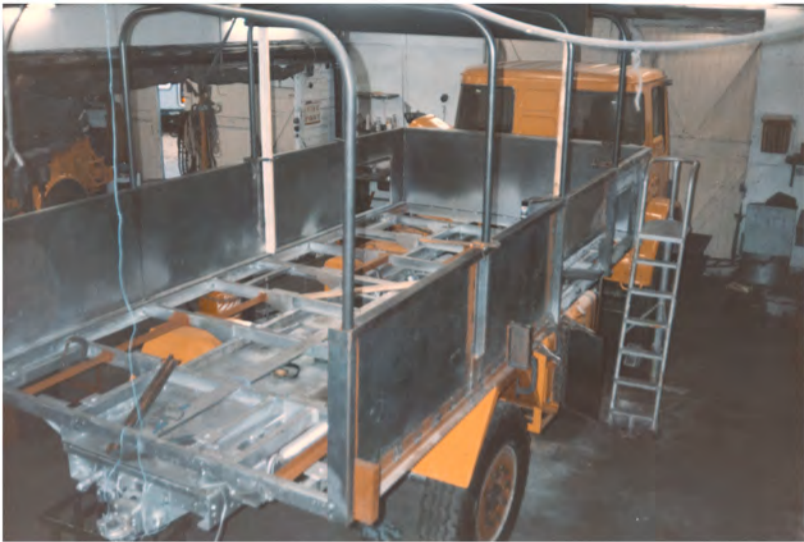
Hoop frames for tilt installed. Access holes for cooking equipment lockers cut out at front of tray. Cook tent pole-carrier, rear mud-guards and jerry-can holders welded in place.
